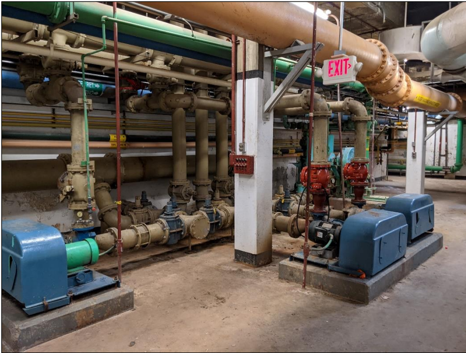
Figure 2-54 Primary Sludge Pumps
