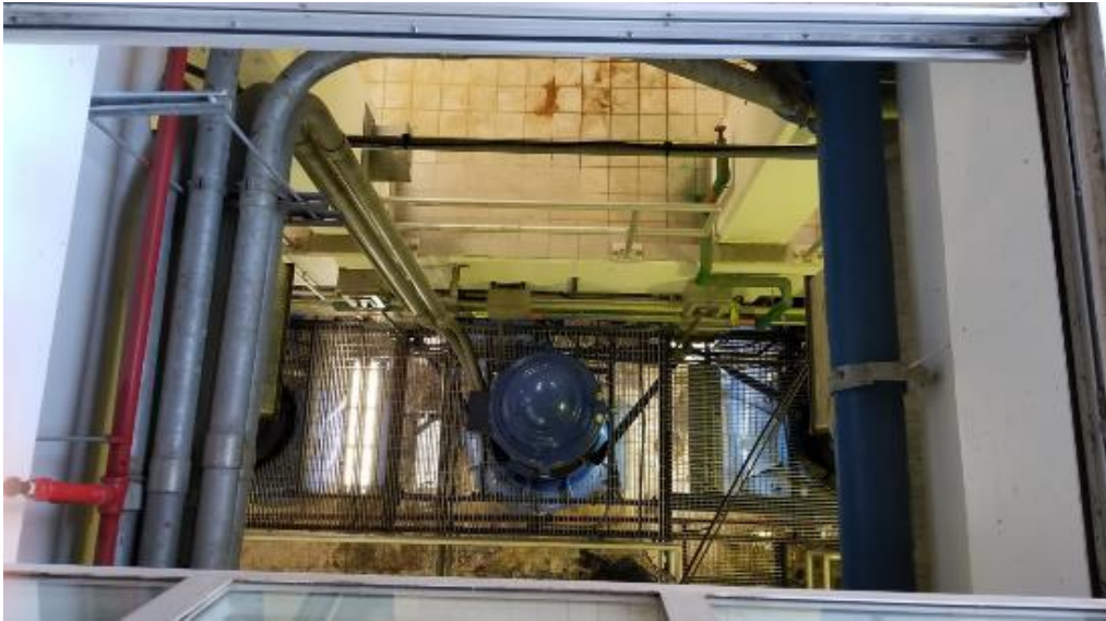
Figure 2-11 Floor Hatches Above Raw Sewage Pumps
