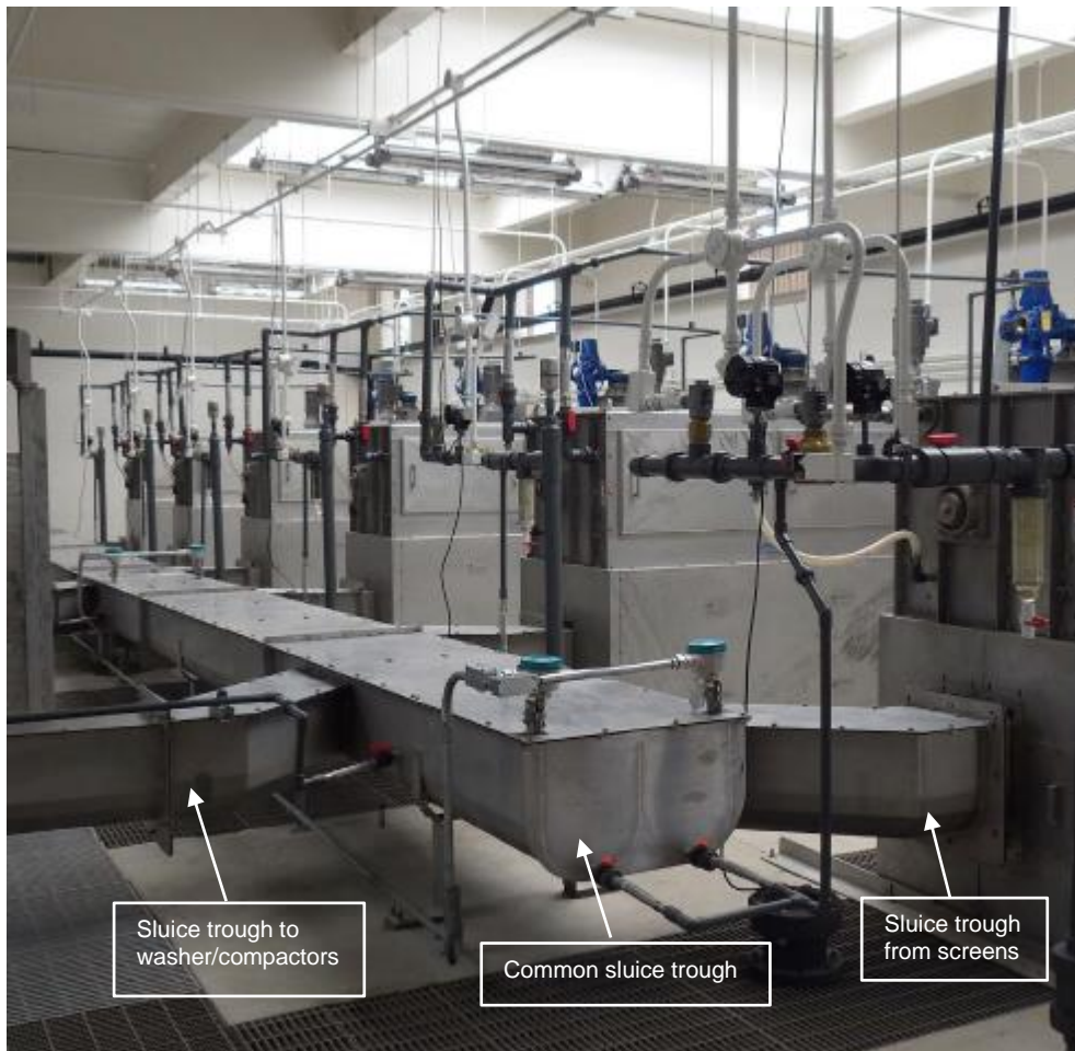
Figure 8-3 Typical Screening Sluice Installation (Courtesy of HydroDyne)
