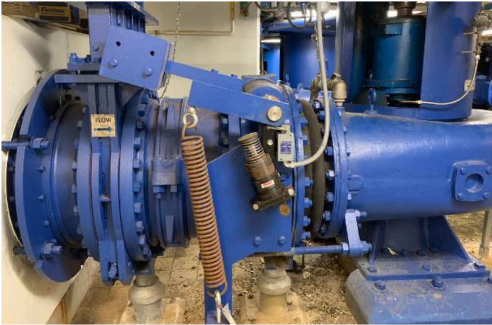
Figure 2-13 Typical Raw Sewage Pump Discharge
