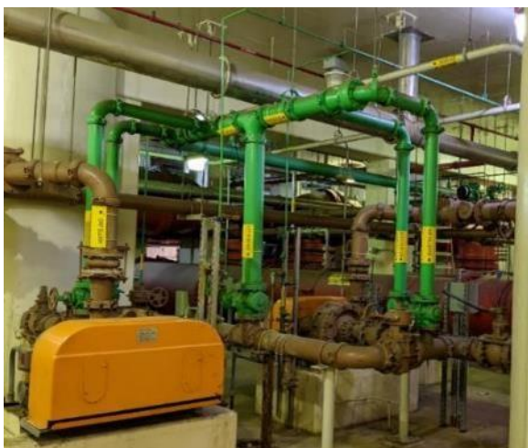
Figure 2-35 Grit Pumps 3 and 4 Interconnection and W3 Flushing Lines
