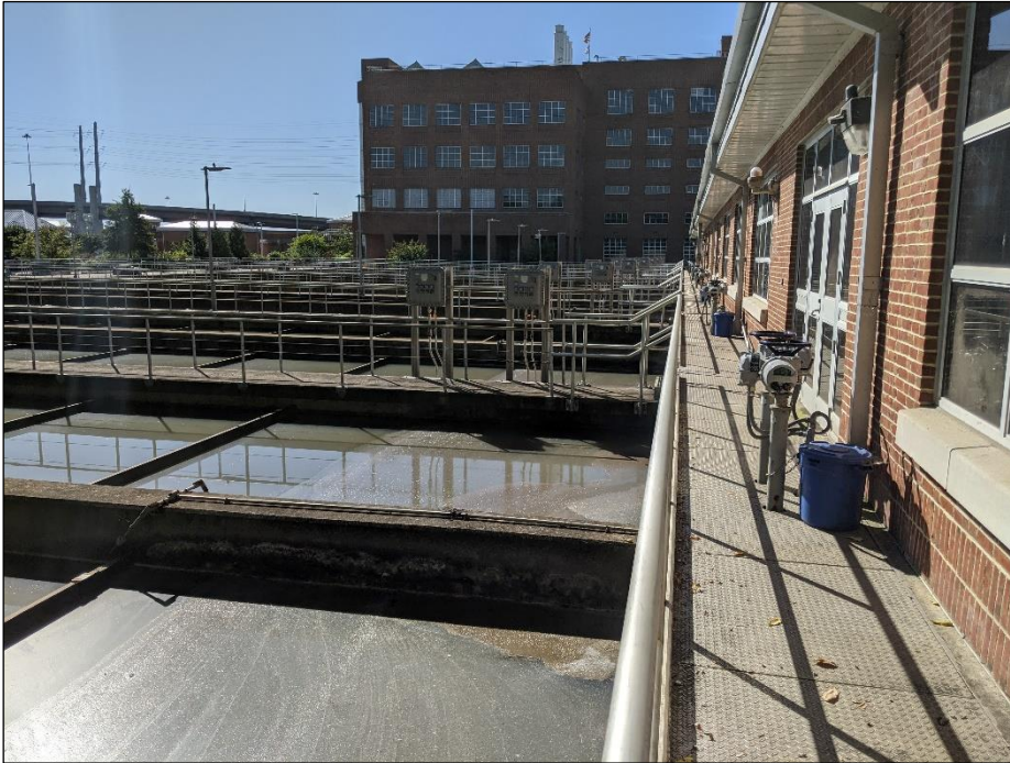
Figure 2-53 Primary Settling Tank Scum Skimmer Electric Actuators
