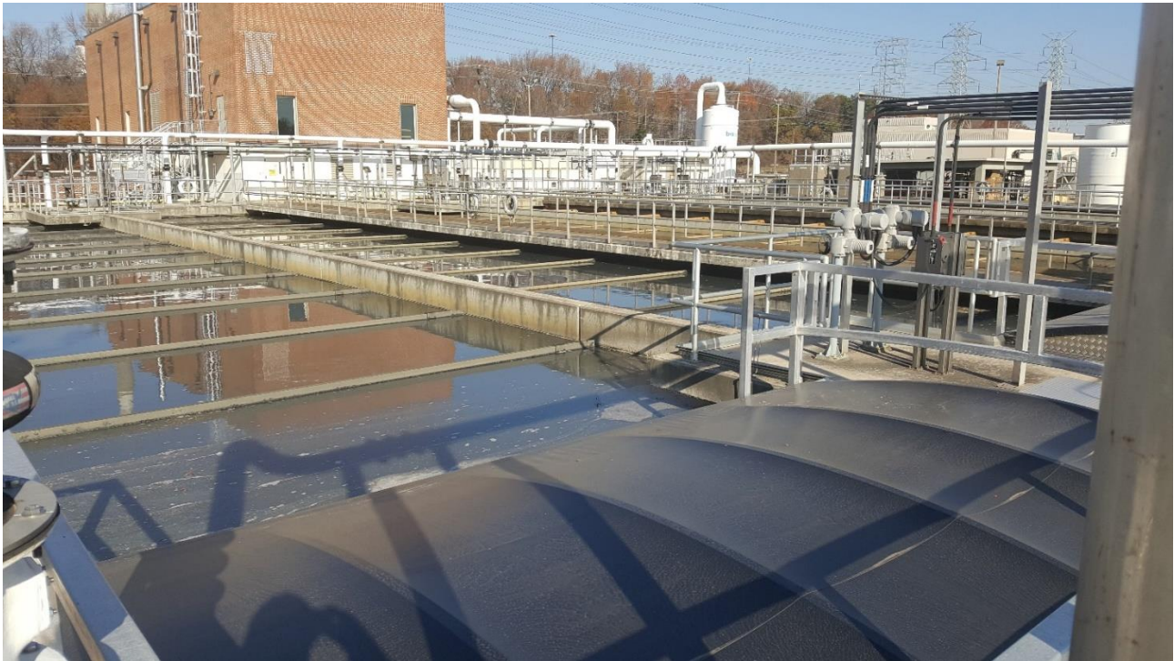
Figure 11-5 Retractable Fabric Covers (Cox Creek WRF, Anne Arundel County MD)
