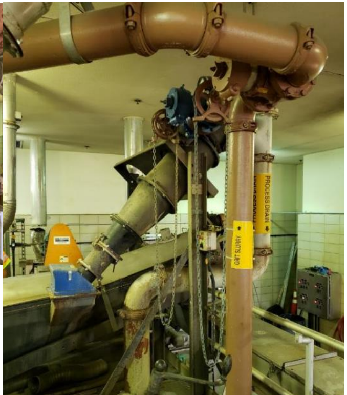
Figure 2-38 Grit Hydrocyclone Unit
