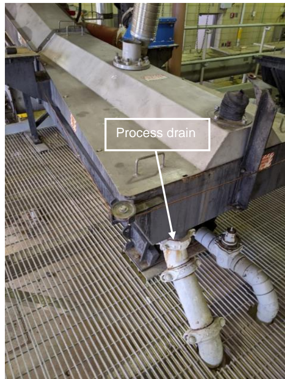
Figure 2-40 Grit Classifier and Process Drain
