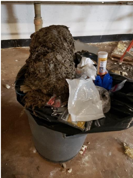
Figure 11-1 Solids Removed from Primary Sludge Pumps
