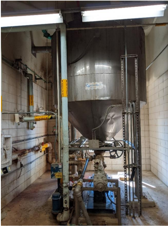
Figure 2-58 Concentrated Scum Tank and Pump
