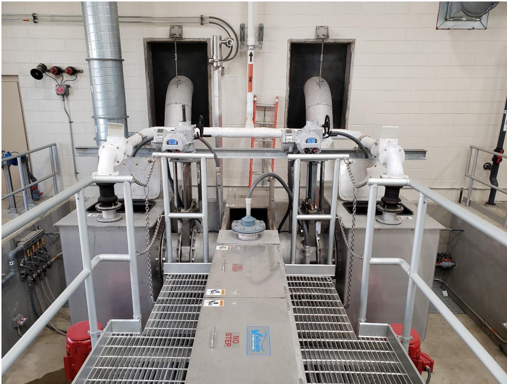
Figure 8-5 Side by Side Washer Compactors Fed From a Central Sluice At The Back River WWTP
