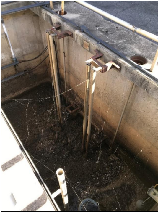
Figure 2-56 Scum Pumping Station
