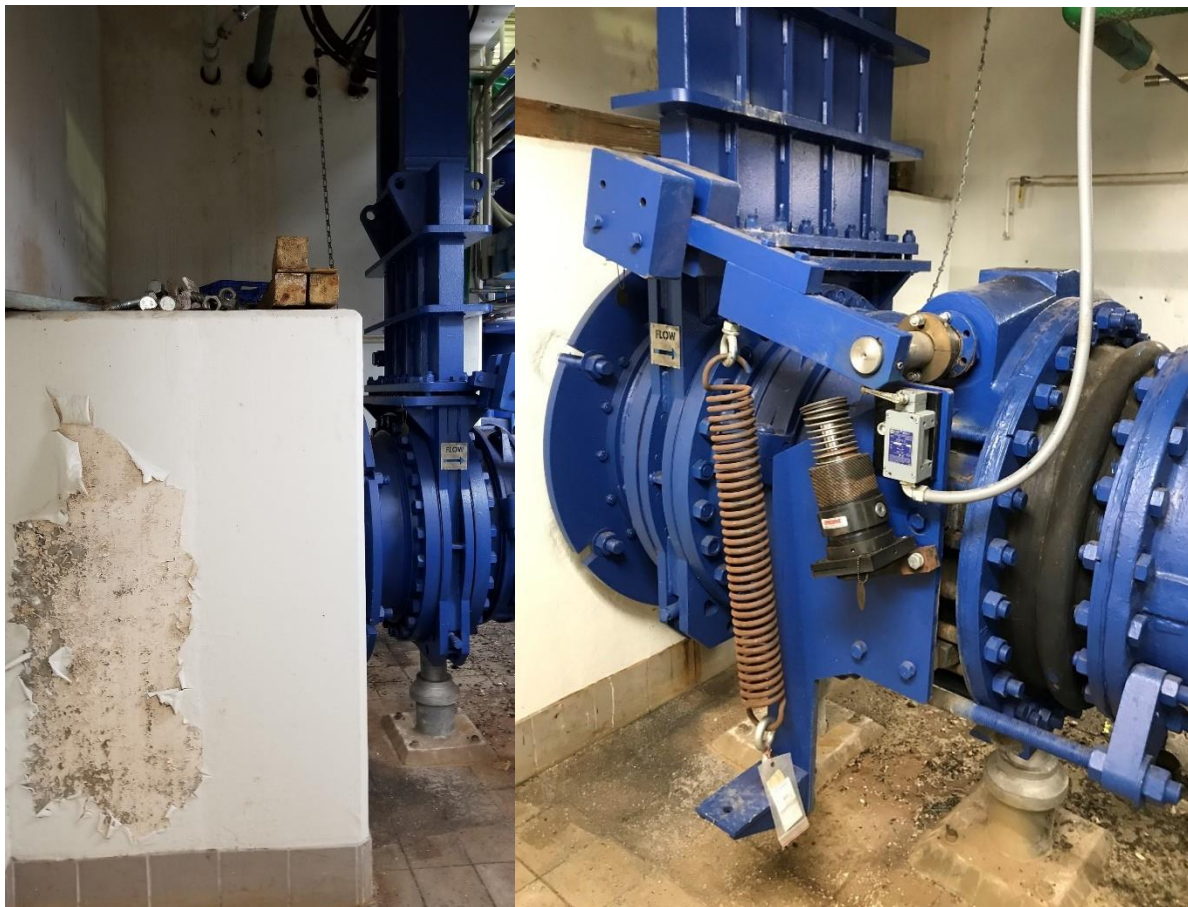
Figure 2-19 Building A Pump Room - South Side discharge conduit (left) and Discharge Piping Arrangement (right)
