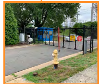
WRRF Site Security and Access Project New gates and guard booths installed and operational in September 2020
