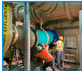
108 to 116 MGD Expansion Project Pumps installed and operational in October 2020
