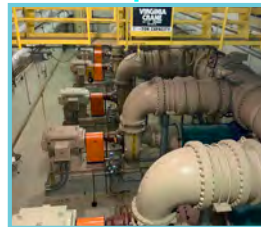
Upgraded Primary Effluent Pumps
