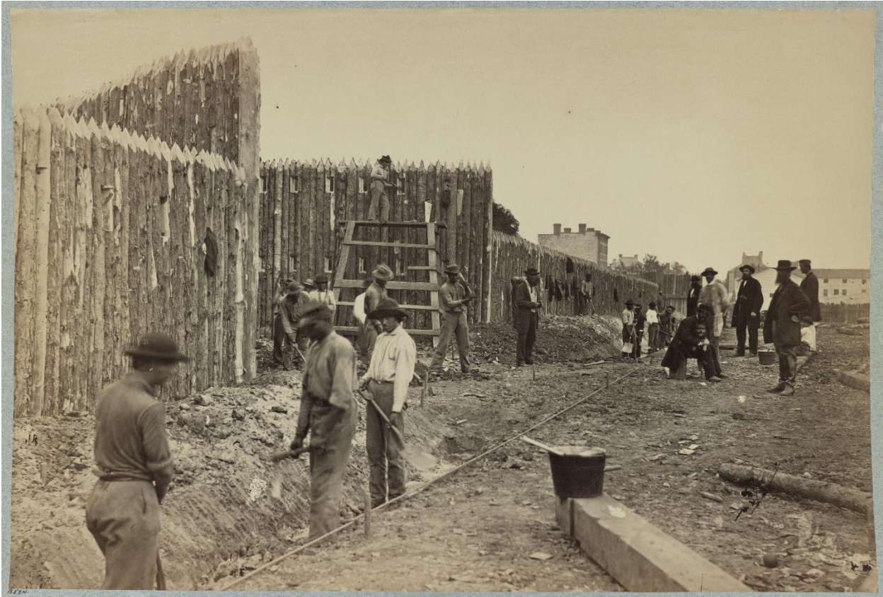
Figure 3 - Building Stockade in Union Occupied Alexandria (Library of Congress Prints and Photographs Division)
